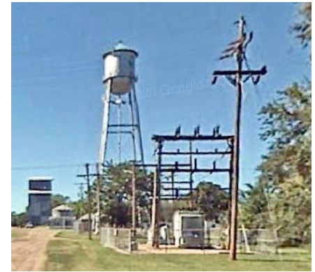
Nickerson Electrical Substation
