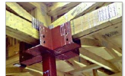
example: Building Code violation
