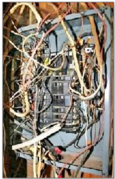
example: Electrical Code violation
